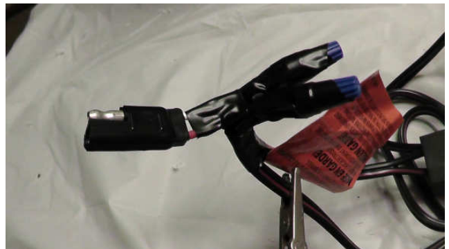
Fig. 19 Wiring after taping
